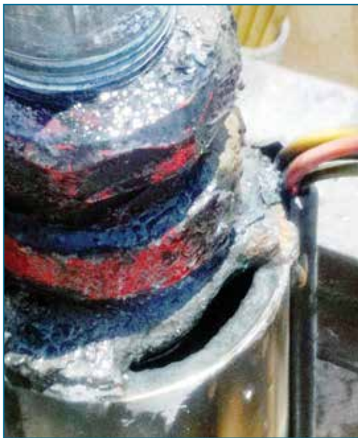
FIGURE 35. Stray electrical currents formed a hole in this submersible pump. Water was forced through the hole in the bottom of the pump, causing the well screen to collapse and the well system to fail. (Source: Mike Prestigiacomio)
