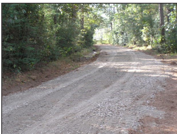
Figure 49. Armoring road surfaces can prevent erosion and improve accessibility. (Photo courtesy of the Texas Forest Service.)
