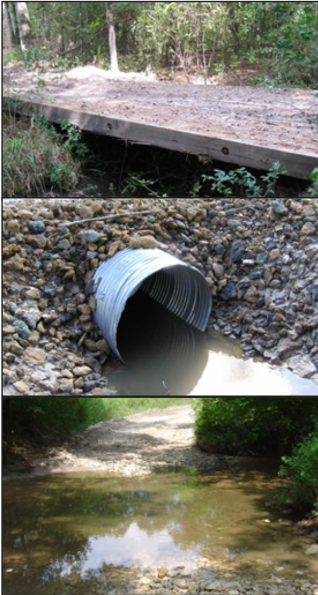
Figure 46. Bridges, culverts, and fords are among the most common types of stream crossings. (Photo courtesy of the Texas Forest Service.)
